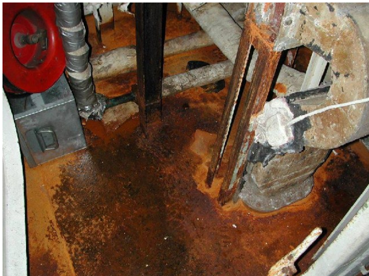
Rusted Deck and Ventilation Equipment Source: www.corrdefense.org
